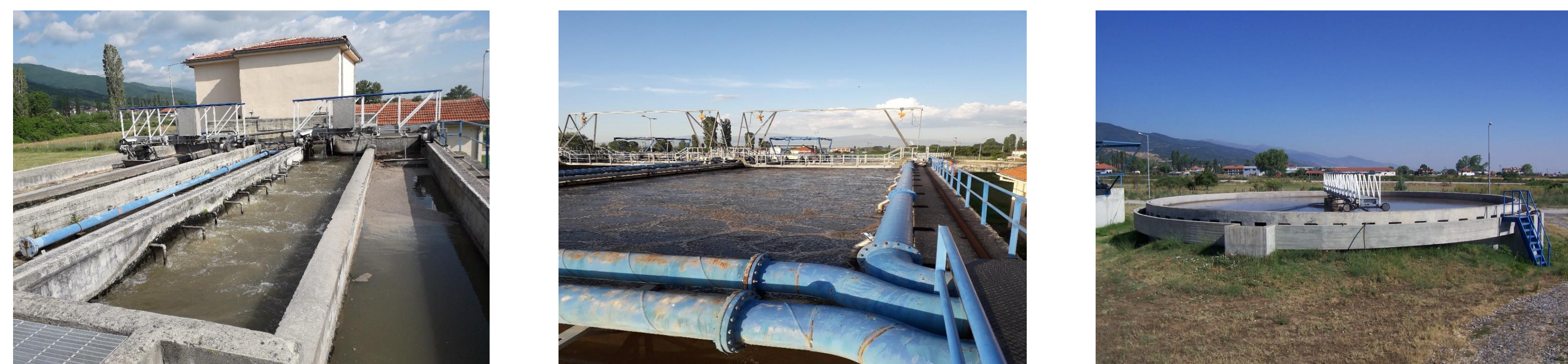
Figure 1: View of some of the Florina WWTP tanks (grit tanks, activated sludge aeration, secondary sedimentation)
